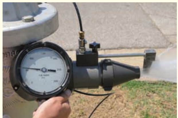
Figure 6 A pitot tube is used on fire hydrants to determine the amount of water that is available for a building.
