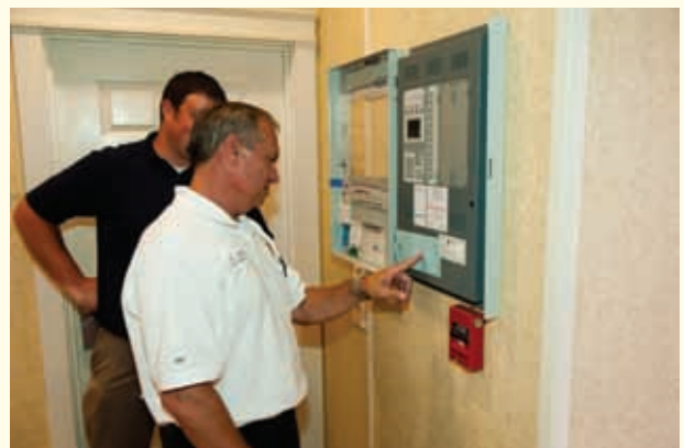
Figure 11 Fire alarm systems and automatic fire sprinkler systems should be at the top of your list when taking into account the building's fire protection features.
