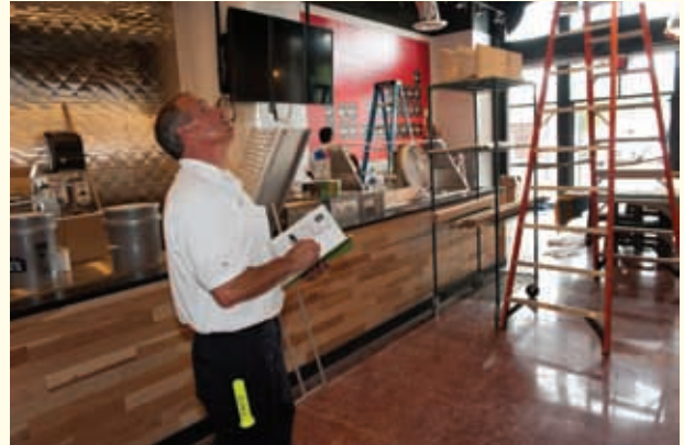
Figure 2 Construction or final inspections are conducted as a building is being constructed on specific building components including sprinkler systems.
