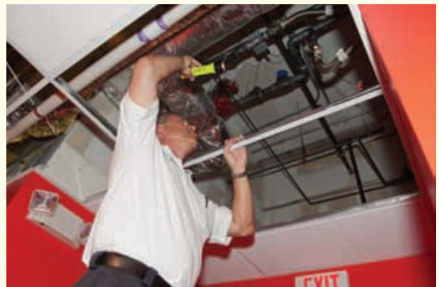
Figure 5 A flashlight is used to check areas behind appliances, rooms where the lighting does not function, and spaces above ceilings.
