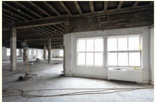
Figure 17 Buildings built long before the fire inspector was born may be renovated multiple times hiding a multitude of construction and fire protection problems. Checking for vertical openings and hidden shafts is a must in older buildings.
